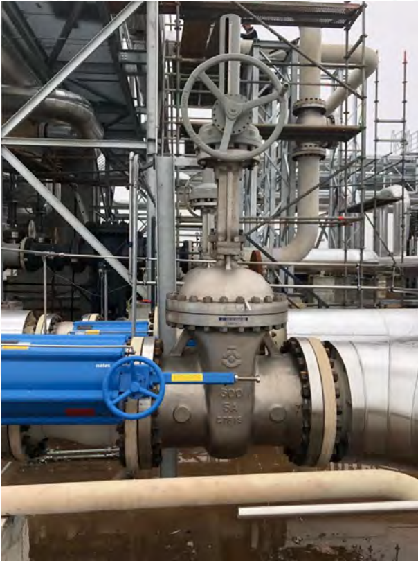
GEOTHERMAL POWER PLANT
