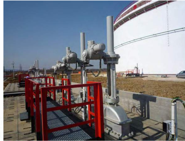
CRUDE OIL TANKS PIPELINE CROATIA
