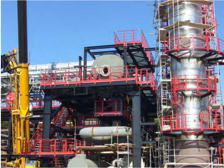
SRU UNIT REFINERY RIJEKA
